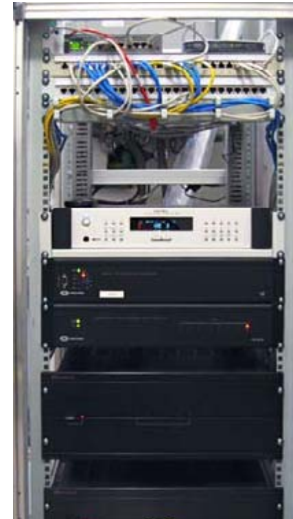
Rack for a relatively small Smart Home system
