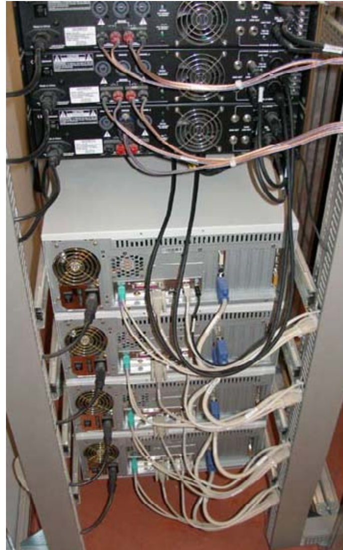
Large rack in a self-contained technology room
