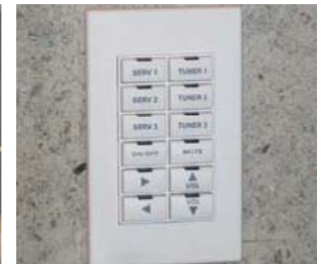
Bathroom with multiroom control panel
