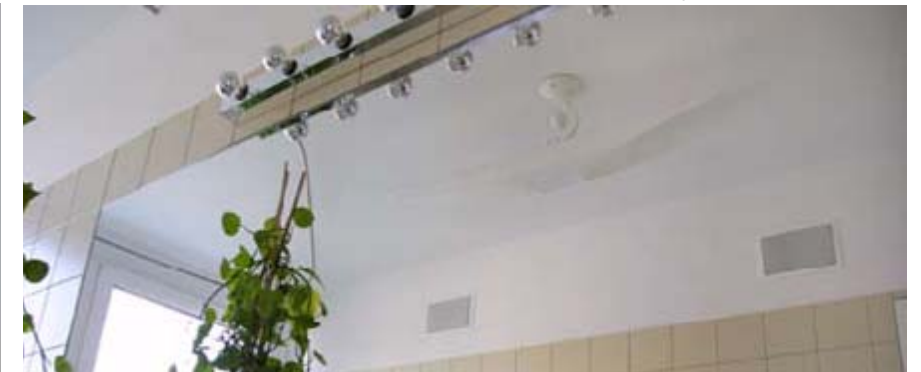
Sunk loudspeakers in the bathroom
